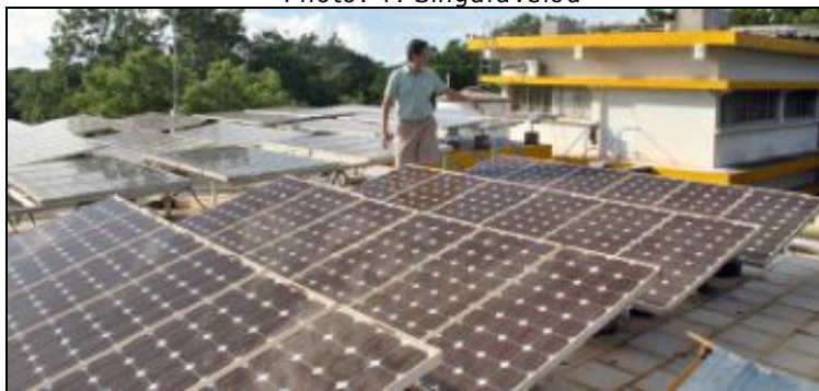
TAPPING SUN: Solar photovoltaic panels at Auroville.
